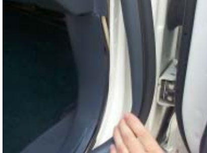
View of DB-25 located on front passenger side, under trim, heading upward toward headliner. Note: power cable will go through firewall towards battery.
